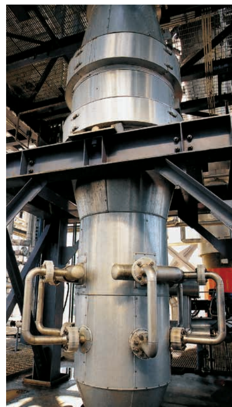
Ammonium nitrate neutraliser
