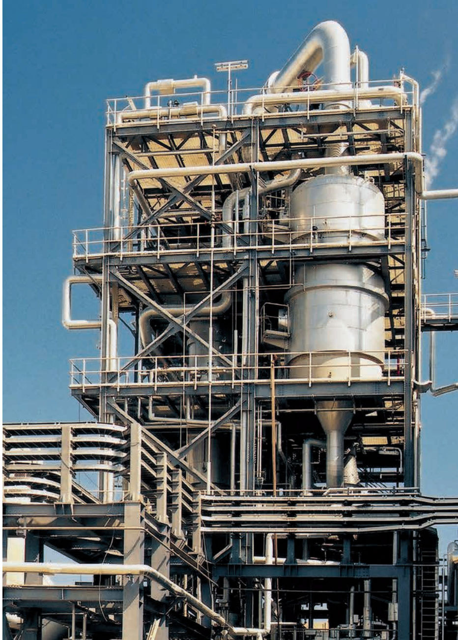
Ammonium nitrate vacuum neutralisation and evaporation unit for Enaex S.A. in Mejillones, Chile. Capacity: 1,060 t/day AN solution (92/96 wt.% AN)
