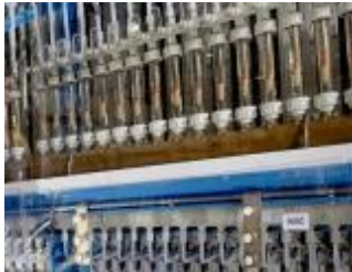
Energy storage Redox-flow
