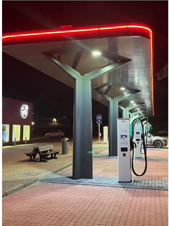
Carports and charging stations, Denmark
