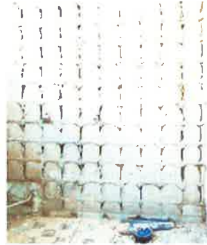
Photo courtesy of the manufacturer. The adhesive strips are applied to the substrate.
