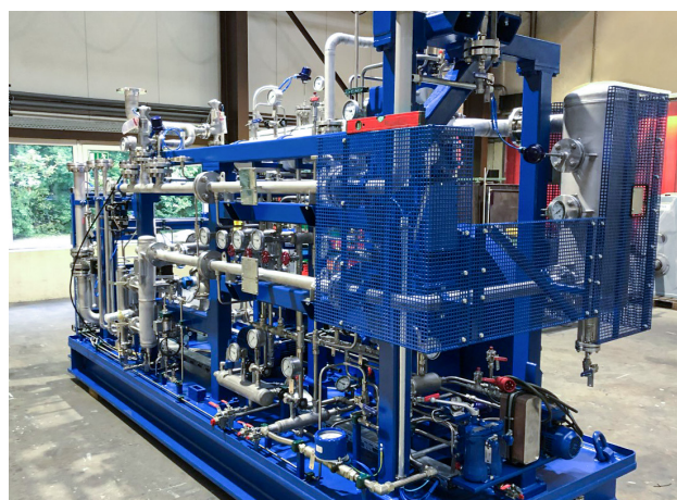
Fig. 4: Compressor for a CO 2 -recovery system.
